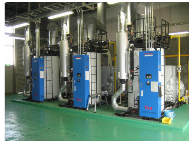
Boilers at the Hikone Plant powered by city gas
