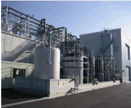
New wastewater treatment plant
