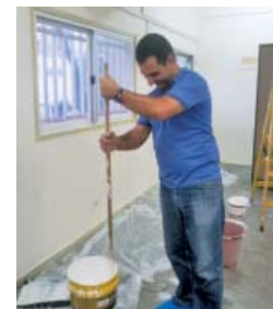
Employees volunteering time to help with the renovation (Dainippon Screen Israel Ltd.)
